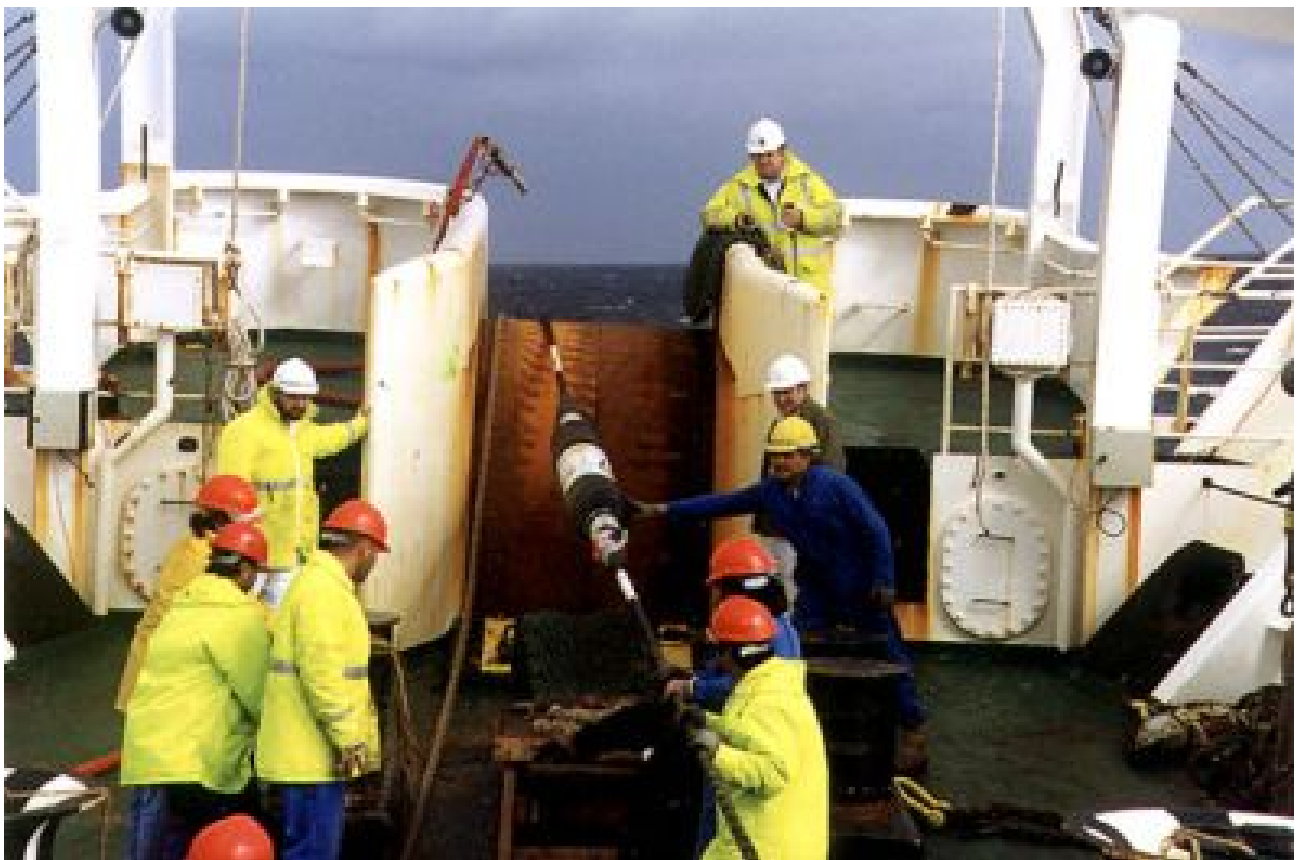
Figure 2: Deployment of a Repeater
